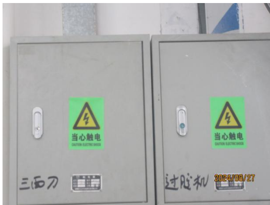
16.Warning sign marked on electricity box.JPG
