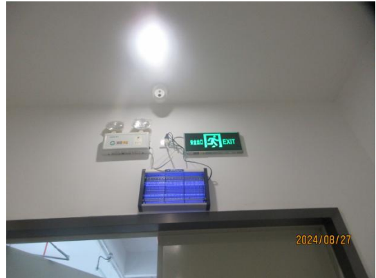
11.Exit sign & emergency light.JPG
